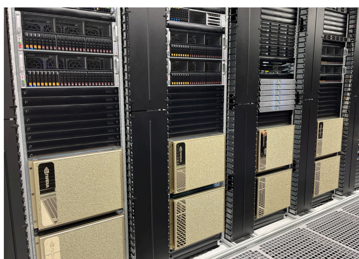
Our AI Data Center with NVIDIA DGH H100 Basepods.
